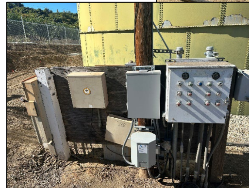
Electrical mounted on Plywood, Undersized Pumps/Panels, Reduced Capacity
